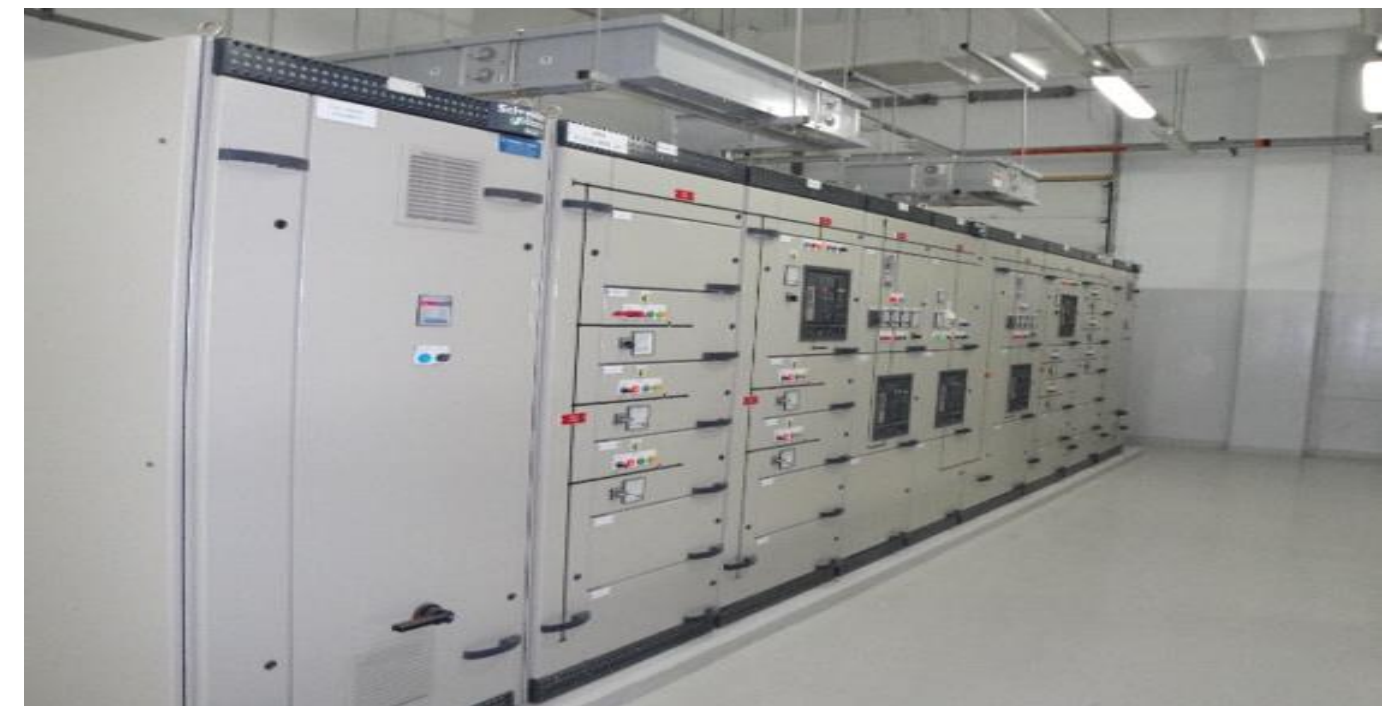
Typical LV Main Distribution Board
